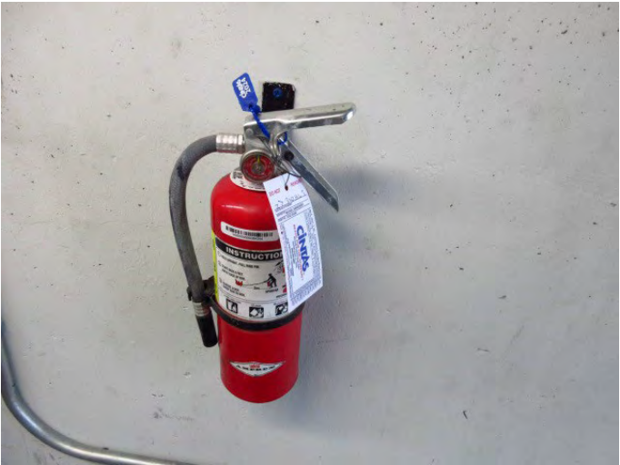
VIEW OF TYPICAL FIRE EXTINGUISHER
