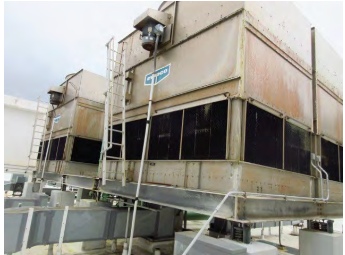
VIEW OF COOLING TOWERS
