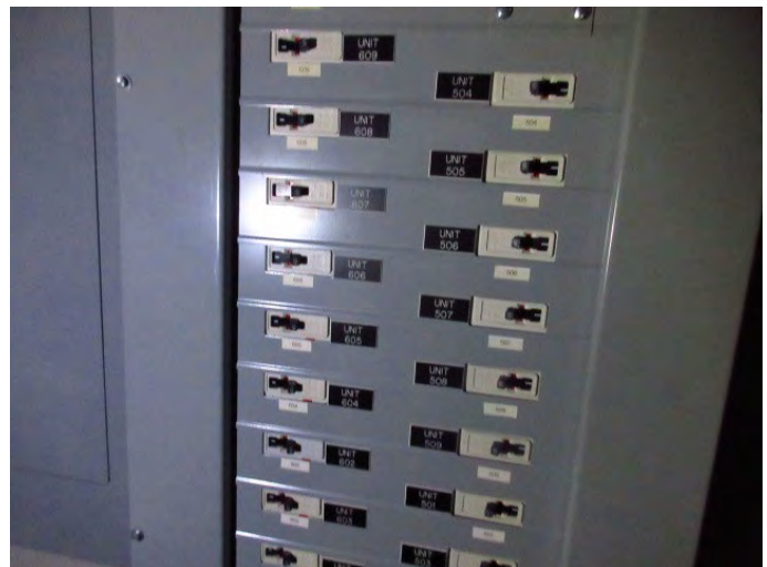
VIEW OF ELECTRICAL EQUIPMENT
