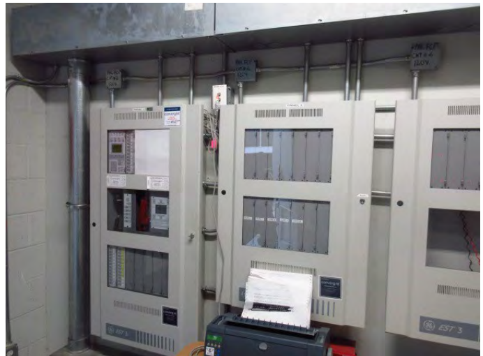
VIEW OF CENTRAL ALARM PANEL
