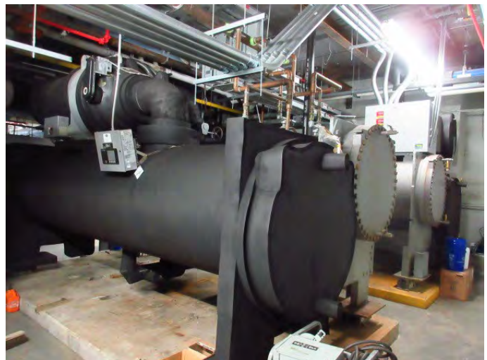
VIEW OF CHILLERS
