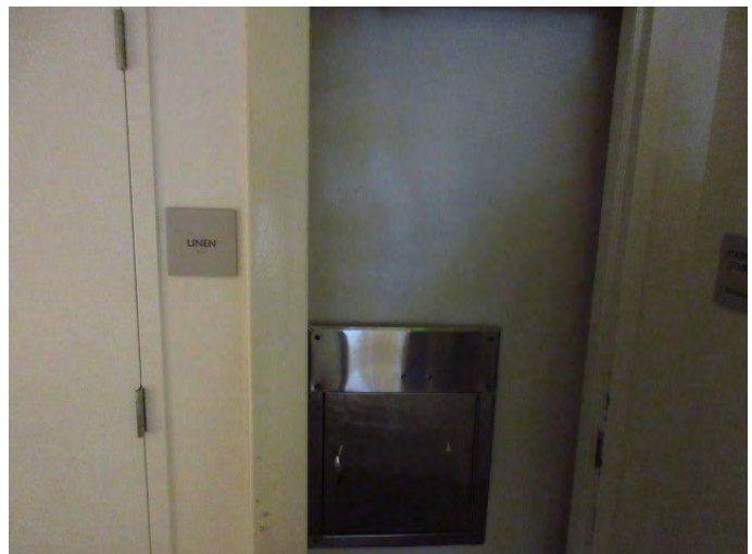
COMMON AREA INTERIOR – LINEN CHUTE
