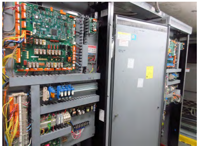
VIEW OF ELEVATOR EQUIPMENT
