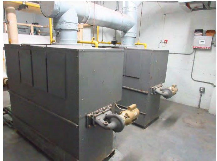
VIEW OF BOILERS
