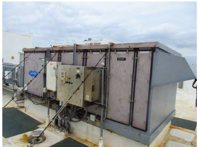
VIEW OF HVAC EQUIPMENT
