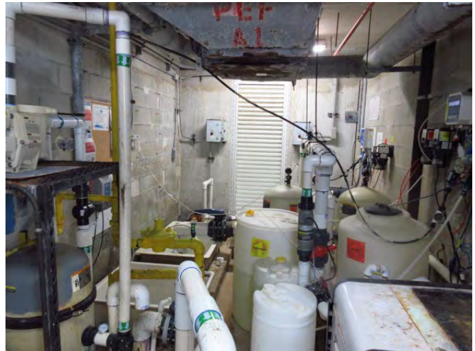
VIEW OF SWIMMING POOL EQUIPMENT
