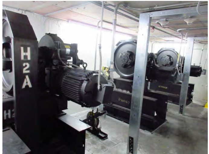
VIEW OF ELEVATOR EQUIPMENT
