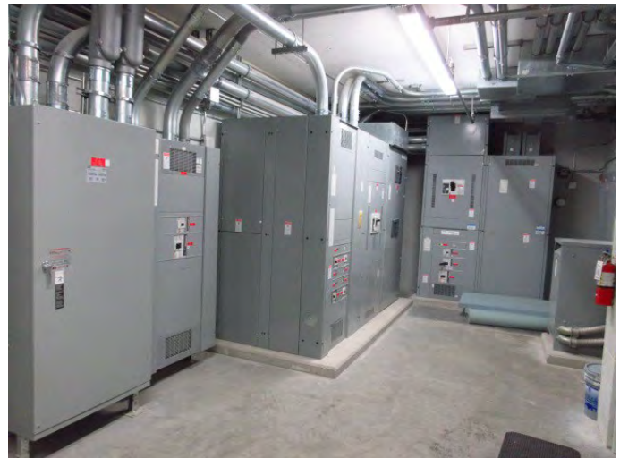
VIEW OF ELECTRICAL EQUIPMENT
