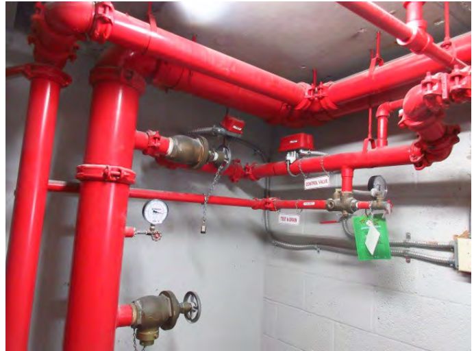
VIEW OF FIRE SUPPRESSION SYSTEM
