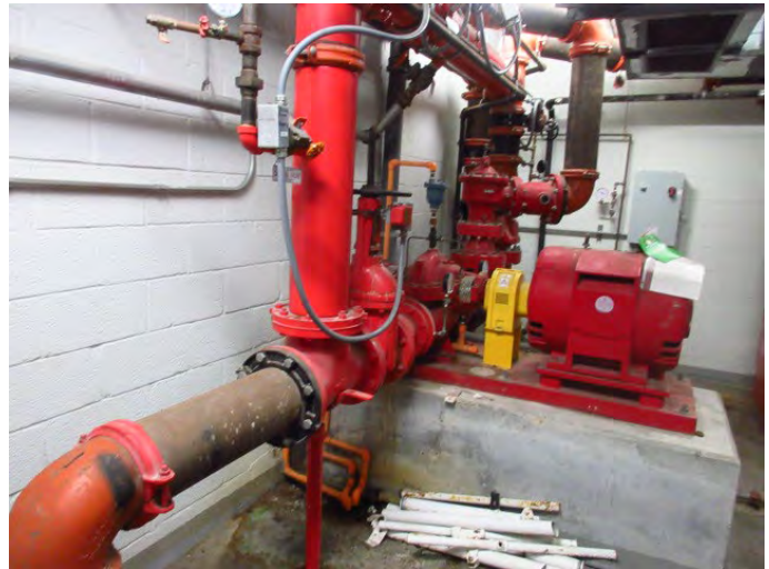
VIEW OF FIRE SUPPRESSION SYSTEM
