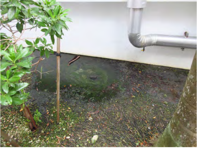
VIEW OF PONDING AT BASE OF BUILDING
