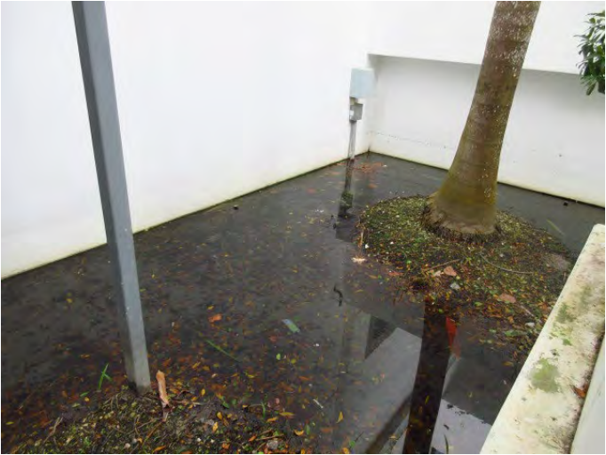
VIEW OF PONDING AT BASE OF BUILDING
